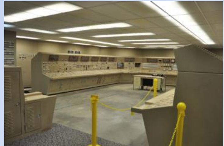
Original Main Control Room
